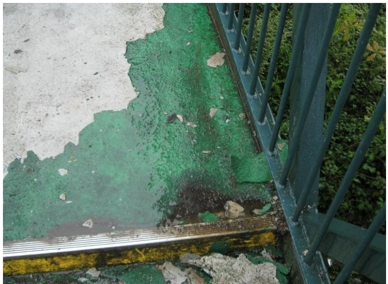
Antislip surfacing lifting
